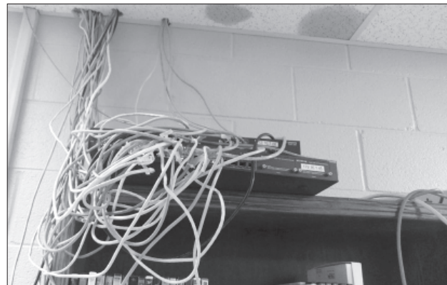
FIGURE 6-4 CABLING AT DALHART JUNIOR HIGH SCHOOL NOVEMBER 2016
